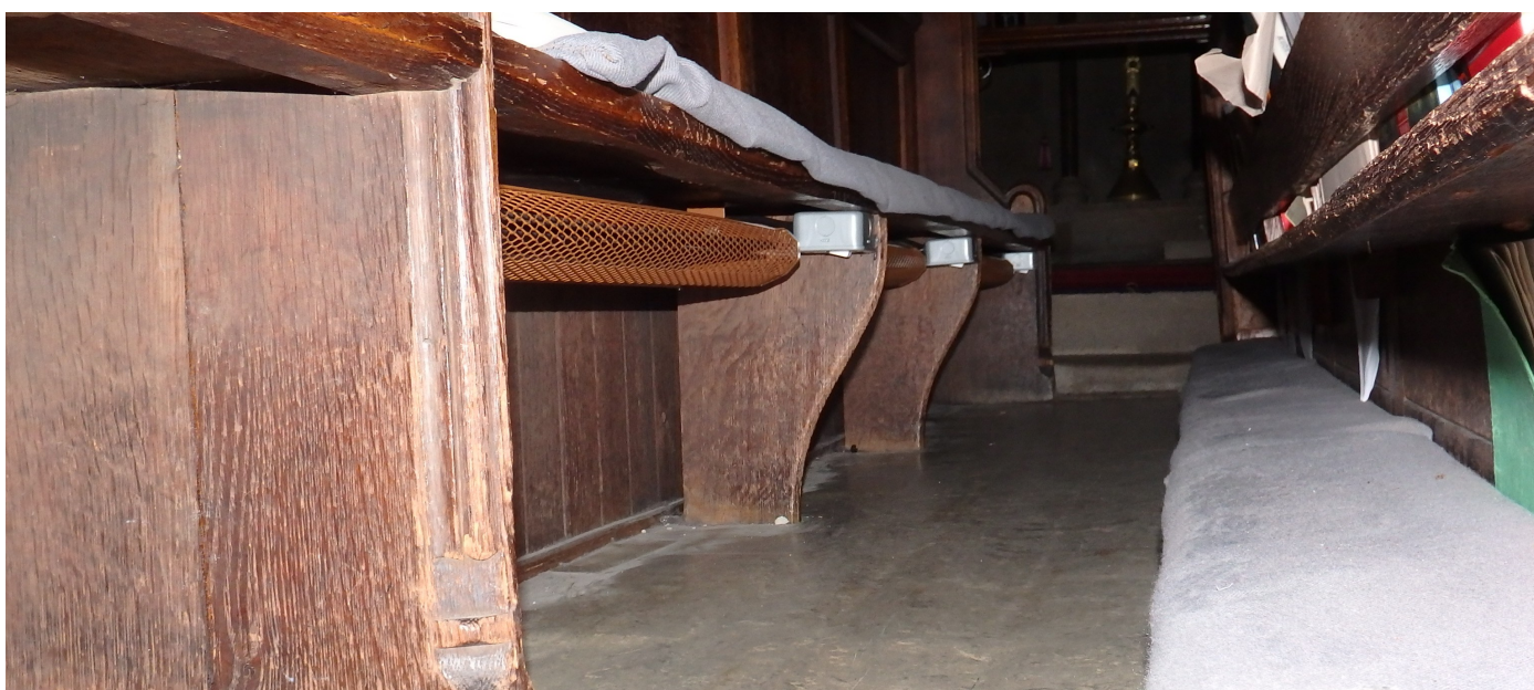
Under-pew heaters in the choir stalls. There is a switch next to each heater allowing the seat occupant to control the individual heater, with a master switch for each side of the chancel.
