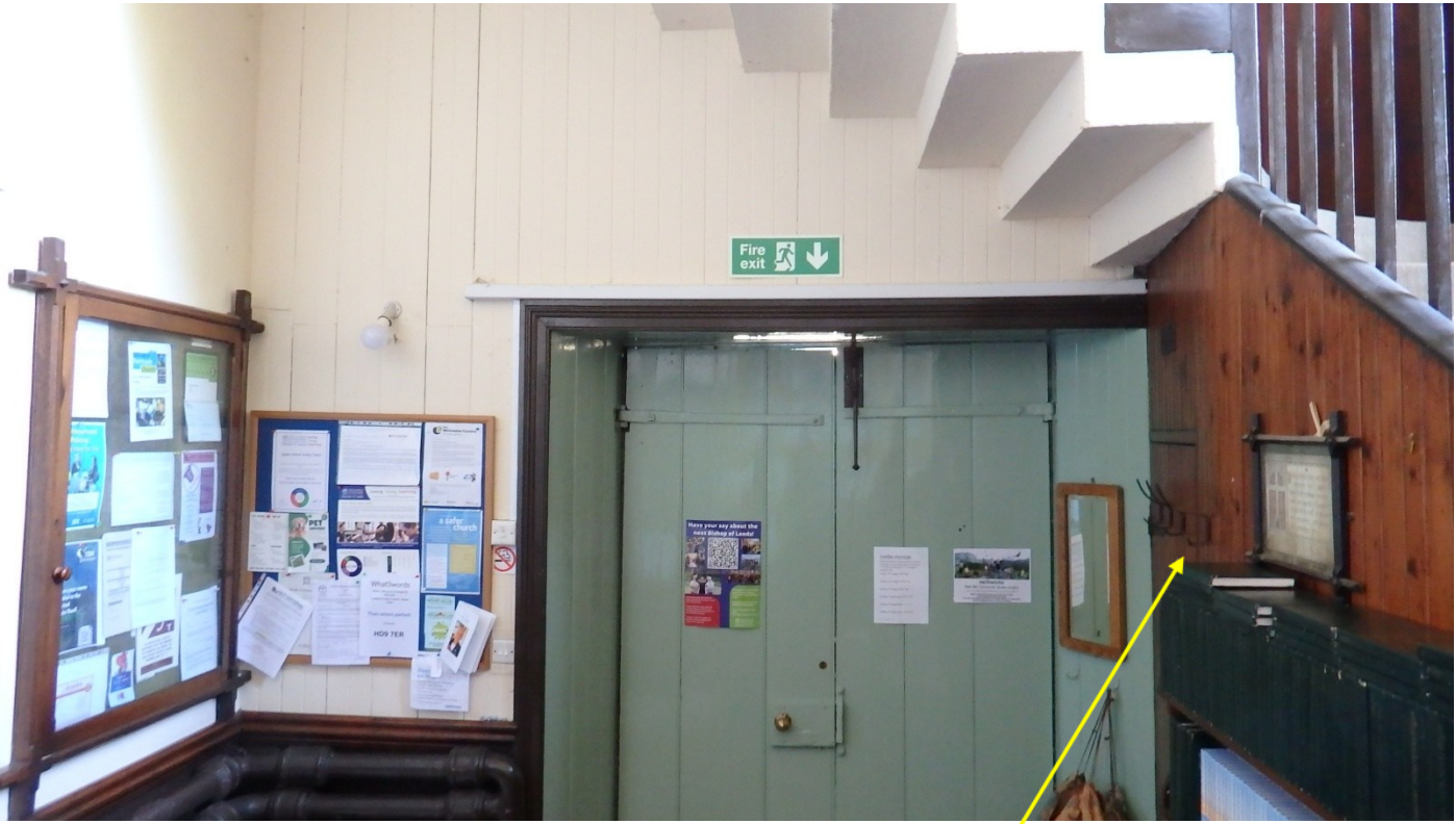
The mains supply distribution is in the compartment under the stairs behind this door.
