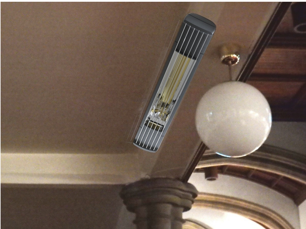
Photograph as above, but showing the typical positioning of the heaters in Zones 1 and 3 of ARC's diagram. Note that these heaters will be white finish to most closely match the painting of the beams. (These heaters are available only in white or black finishes)
