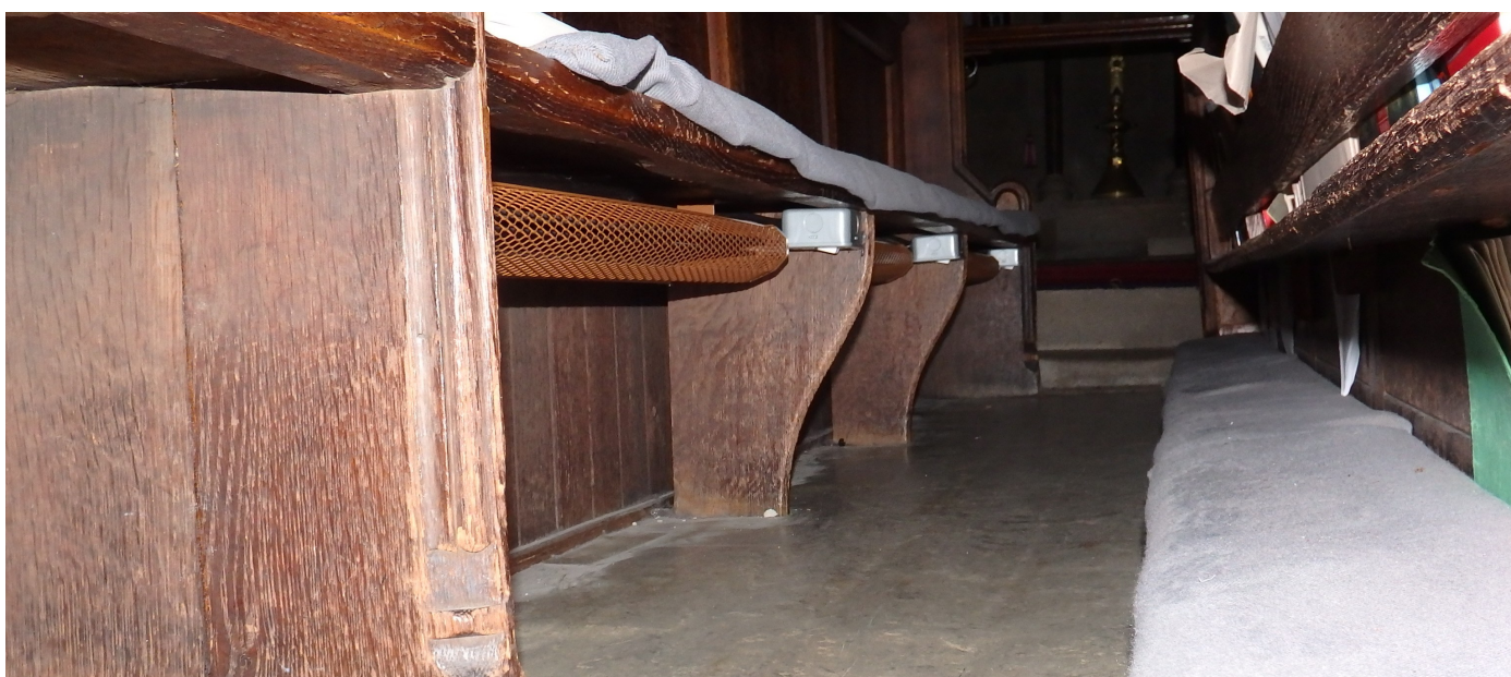
Under-pew heaters in the choir stalls. There is a switch next to each heater allowing the seat occupant to control the individual heater, with a master switch for each side of the chancel.
