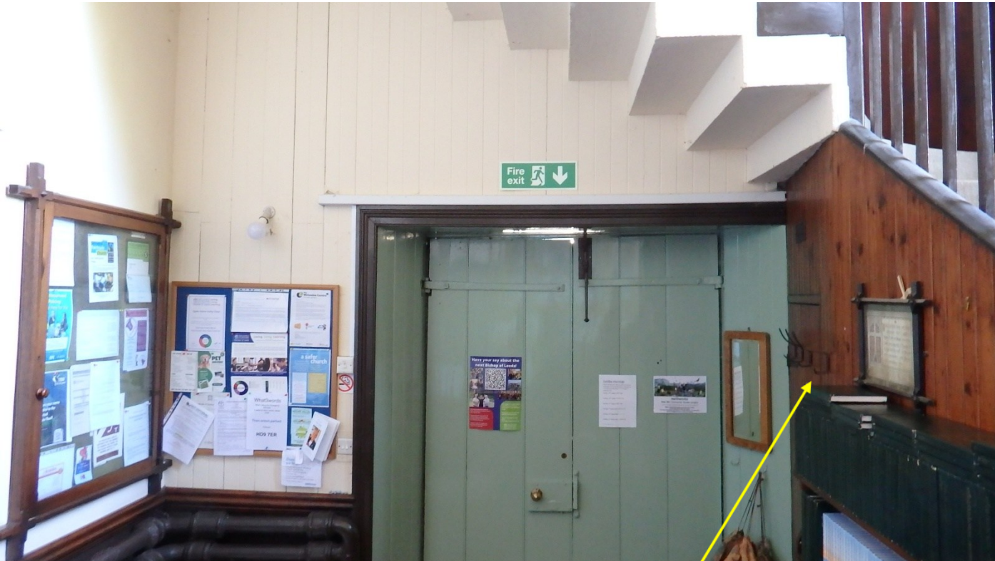
The mains supply distribution is in the compartment under the stairs behind this door.
